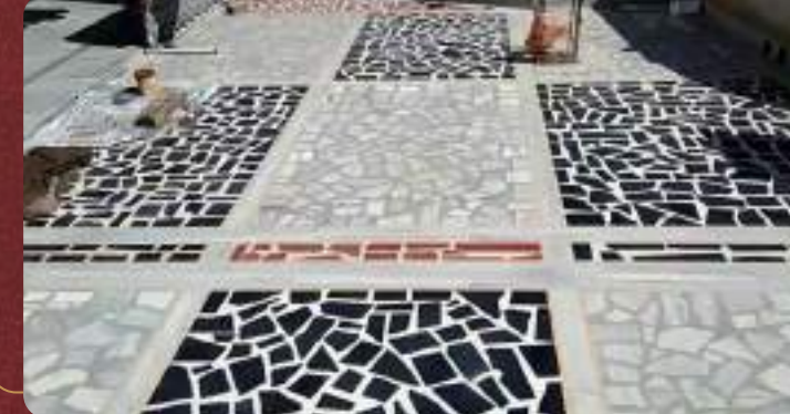
The building roof will be finished with water proofing treatment in brick bat coba with Cement finish / Tukda Tiles China Mosaic finish.
